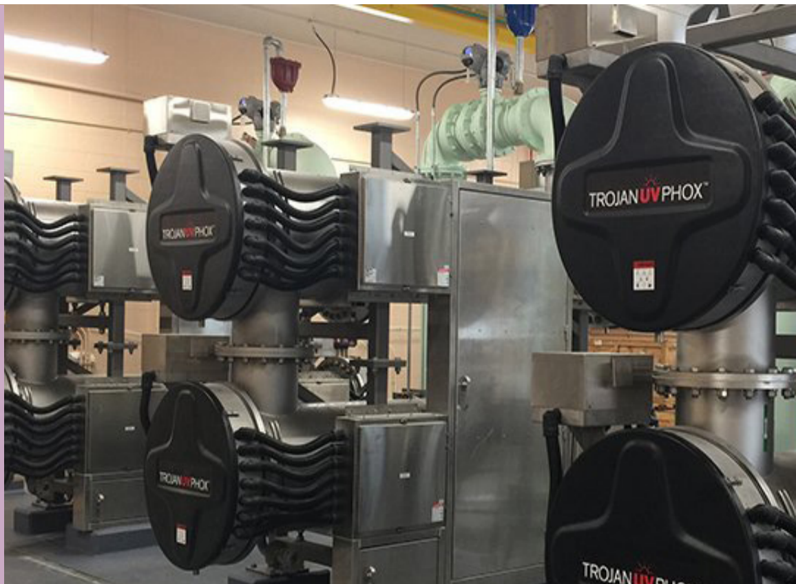
Image: St Anthony Village is the 35th public water system in North America to specifically treat 1,4 Dioxane using Advanced Oxidation with UV-Peroxide. The six (6) Trojan UVPhox Reactors each contain 144 low-pressure high-output UV lamps. The overall system can remove more than 99% of 1,4 Dioxane at Peak Flow Conditions of 3,000 GPM. Source: www.health.state.mn.us (August 2017)
