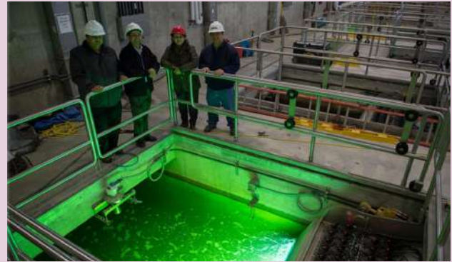
▲ UV treatment process at Chicago wastewater plant.
