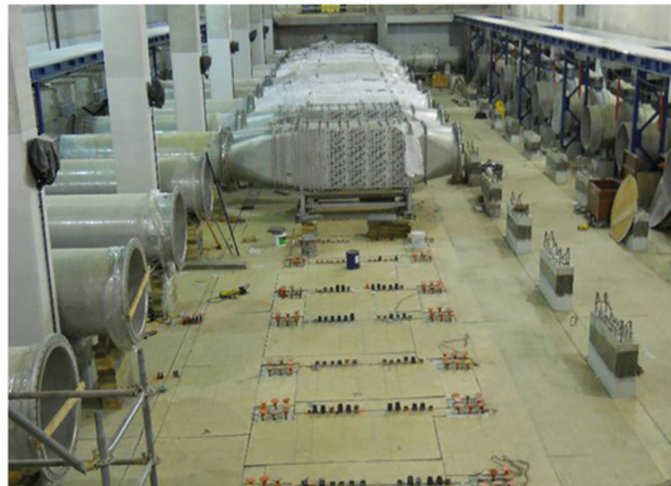
9 of the 56 UV reactors are installed. Every reactor will hold 210 UV lamps
